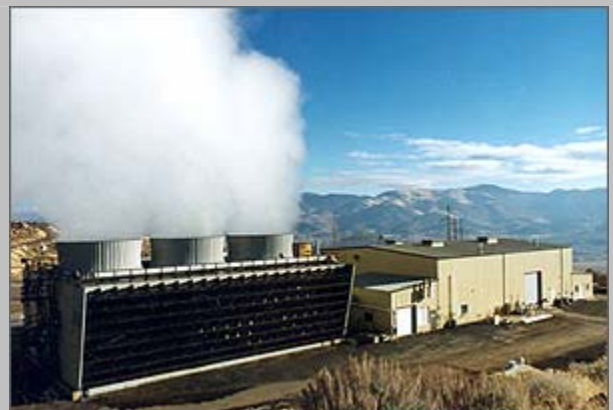
A geothermal power plant in Washoe, NV Photo: U.S. Department of Energy, Office of Renewable Energy and Energy Efficiency
