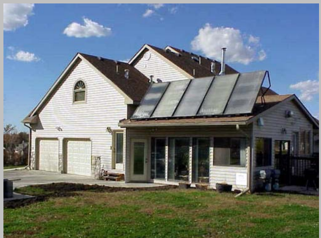
This residence in Missouri has five 4' X 8' solar panels installed. The panels, together with the solar green house, provide 40%-50% of the heating needs for the home during the winter and a year-round supply of domestic hot water. Photo: Ken Riead/NREL
